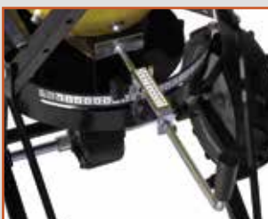
Gate opening control
